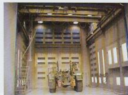
Full Floor Reclaim Blast Room (Retro-fit Vacuum Floor to Mechanical Screw Design)
